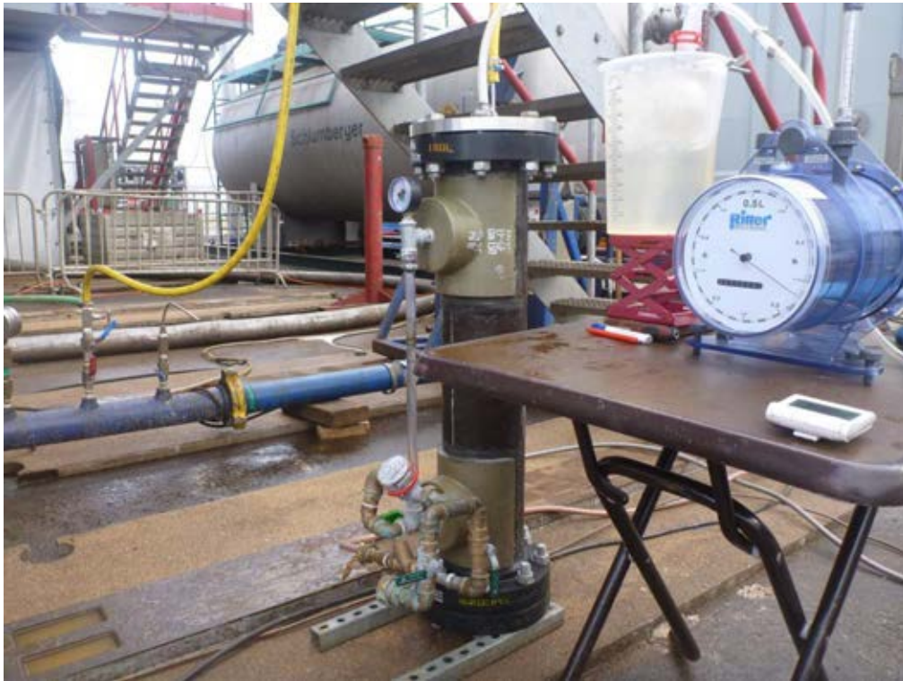
Figure 1: Degasser at the well Honselersdijk Gt 1
